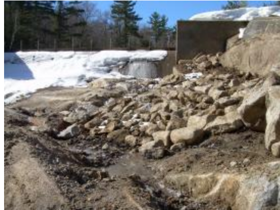
View of existing ledge stream channel looking east towards the spillway of the Gregg Lake Dam.
