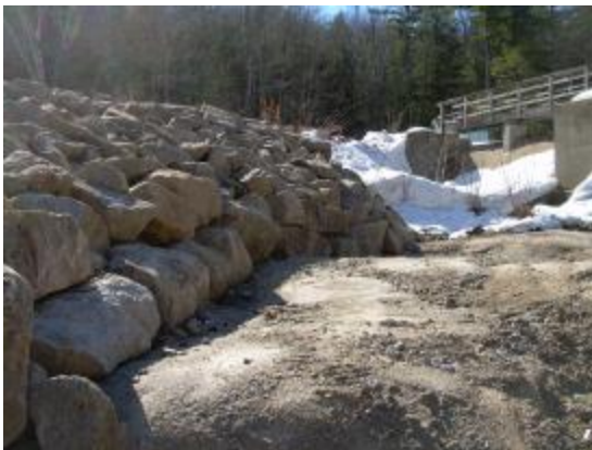
View of the toe of slope from the stream channel along the upstream south embankment along White Birch Point Road.
