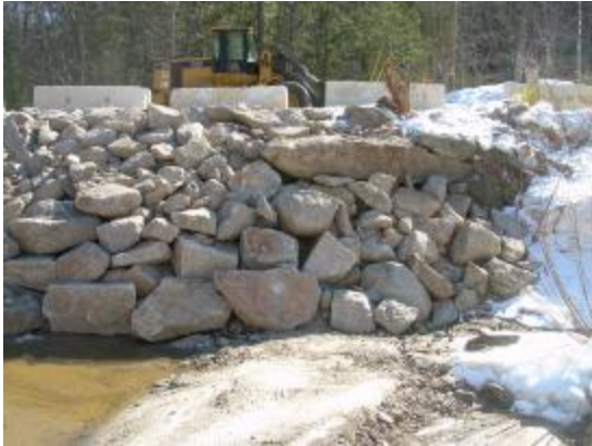
Stone fill tie-in with the existing rock retaining wall on the upstream south embankment along White Birch Point Road.
