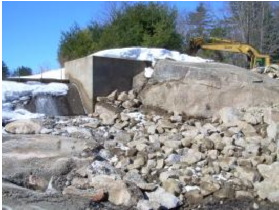
View of the existing ledge and stone fill installation near the north end of the Gregg Lake Dam.
