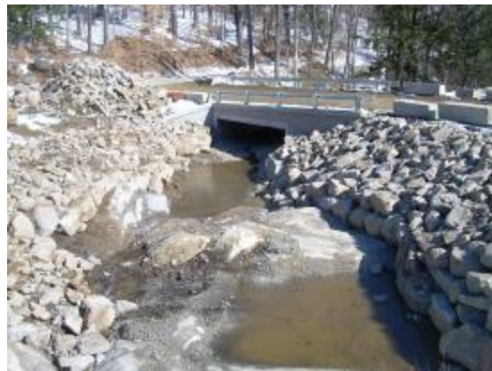
View from the south end of the spillway on Gregg Lake Dam looking downstream towards the new bridge.
