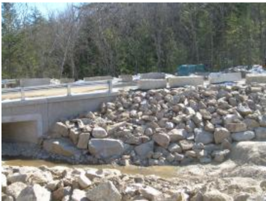
Partial view of the upstream south embankment stone fill installation near the south end of the new bridge.
