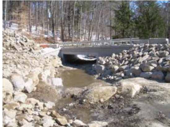
View of the existing stream channel looking downstream towards the north east.
