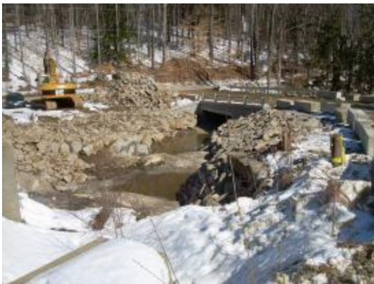
View from the south end of Gregg Lake Dam looking downstream towards the new bridge.
