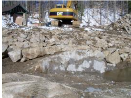
Remaining portion of large area of ledge (view looking north) that would have obstructed the flow of water from Gregg Lake Dam.
