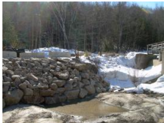
Partial view of the upstream south embankment stone fill installation near the south end of the Gregg Lake Dam.
